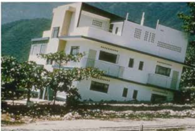
Figure 1: Large differential settlements due to liquefaction under a building (without obvious structural damage) during the Caracas Venezuela 1967 earthquake ( M = 6.5 )
